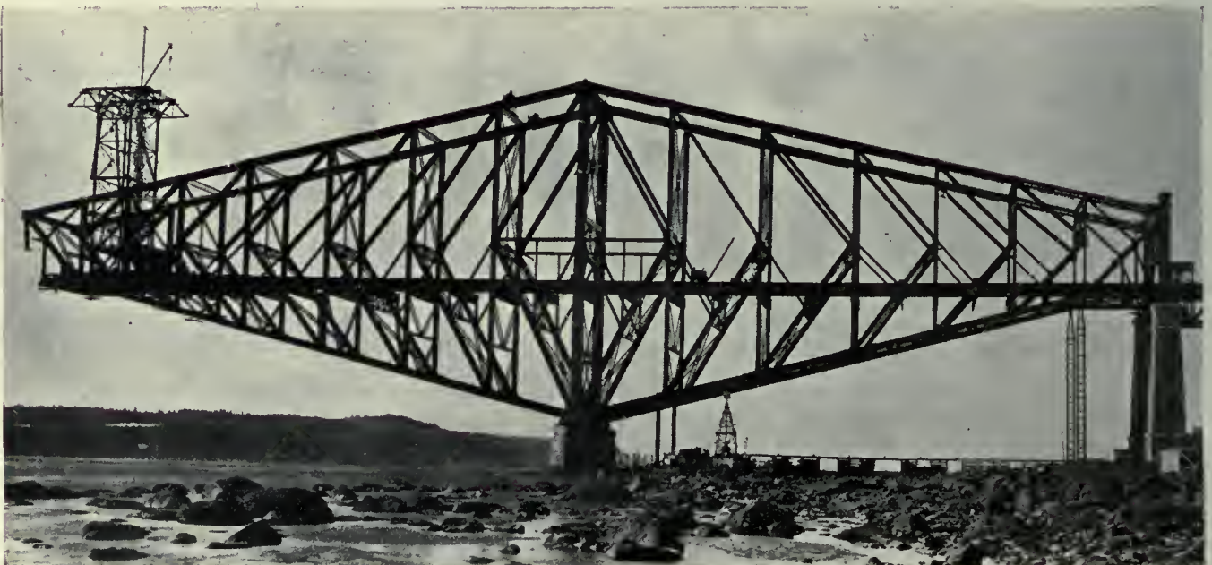
Fig. 4.—Completed north anchor and cantilever arm—Traveller being taken down to be used in the erection of the suspended span.
